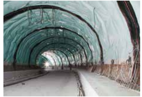
Fig. 26: Road tunnels present a very corrosive environment (de-icing salt and exhaust fumes from traffic).
