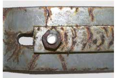
Fig. 8: SCC of a bracket made of the material 1.4301 (A2, 304) after approx. 4 years of use in an indoor swimming pool.
